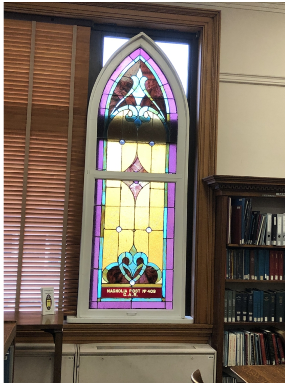
Magnolia G.A.R Post No. 409 Stained Glass Window at its New Home in the Marion Public Library Indiana Room
